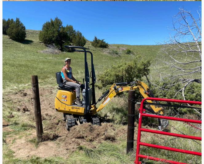
Middle right: a new section of trail leading up to the prairie dog blind, involving cedar stairs and post installation for a railing. May 11, 2024. Photo by Joselyn Andreasen. Bottom right: Joselyn Andreasen working an excavator during trail construction, May 5, 2024. Photo by Jon Garbisch.
