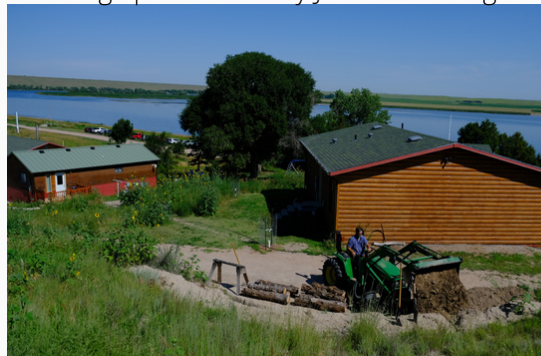
Dru DeLaet installs a cedar retaining wall along the Midge path. Photo by John P. DeLong
