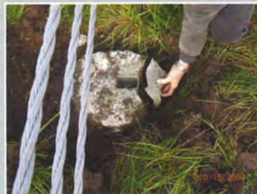
An old post base damaged by severe environmental conditions.
