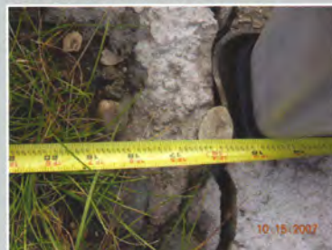
Detail view of the damage.
