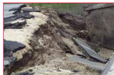
Erosion of a bridge abutment.
